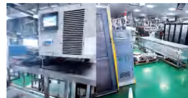
Photovoltaic field-continuous plating Carborundum plating Rectifier
